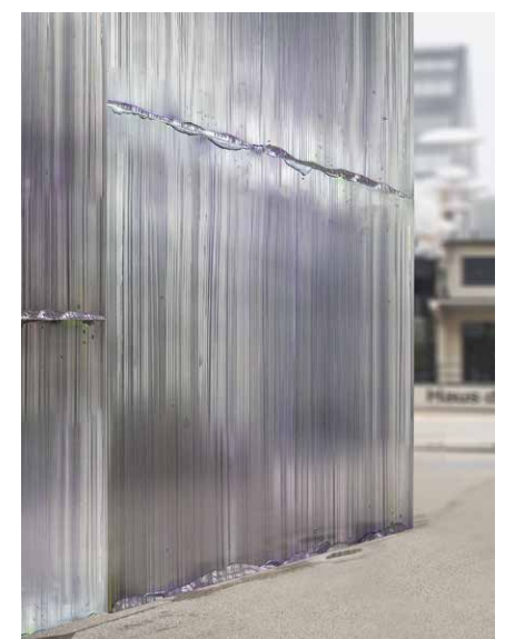
Fig. 4. A mute facade. The marks left from staining discarded sheet metal. Photo © Pa.LaC.E
