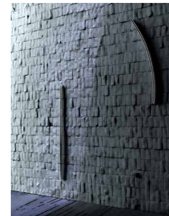
Fig. 3. Using discarded objects together with their ambience. A violent wind enters a dark entry space, through folded sheet metal as air vents. Large solid wall-blocks are reused by milling them for the vents to be embedded. Sunlight passes through reused glass that is dyed. Photo © Pa.LaC.E
